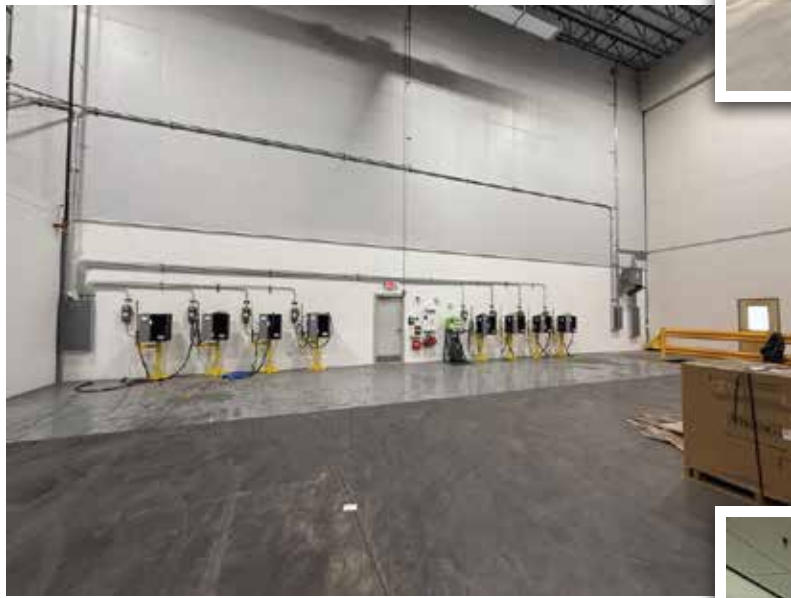
Forklift Charging Stations
